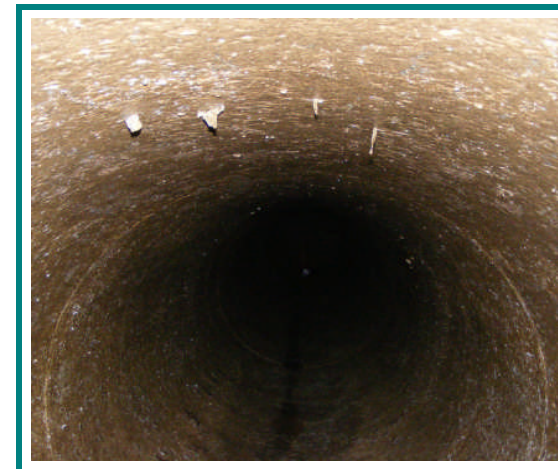
Tunnel #12, minor growth, March 9, 2008
